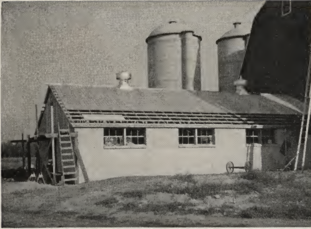
One-story dairy barn constructed as addition to old barn. The concrete floor, lightweight concrete masonry walls and precast window sills and lintels make a serviceable and economical firesafe unit to house the dairy herd.
